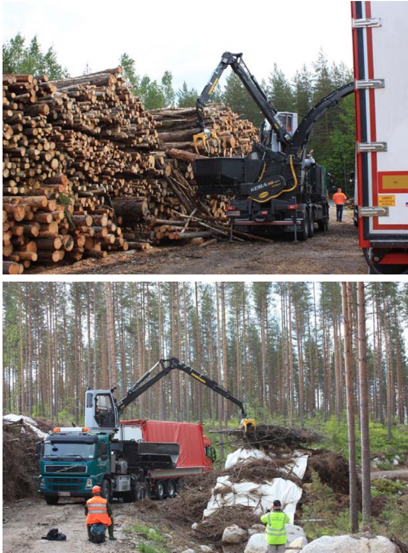
Figure 7 – Chipping non-merchantable roundwood with the Kesla C 860 H hybrid chipper at the wood terminal in Tikkakoski (top) and logging residues (down) at the roadside landing in Uurainen (Photos: Petri Kaksonen/Kesla).
