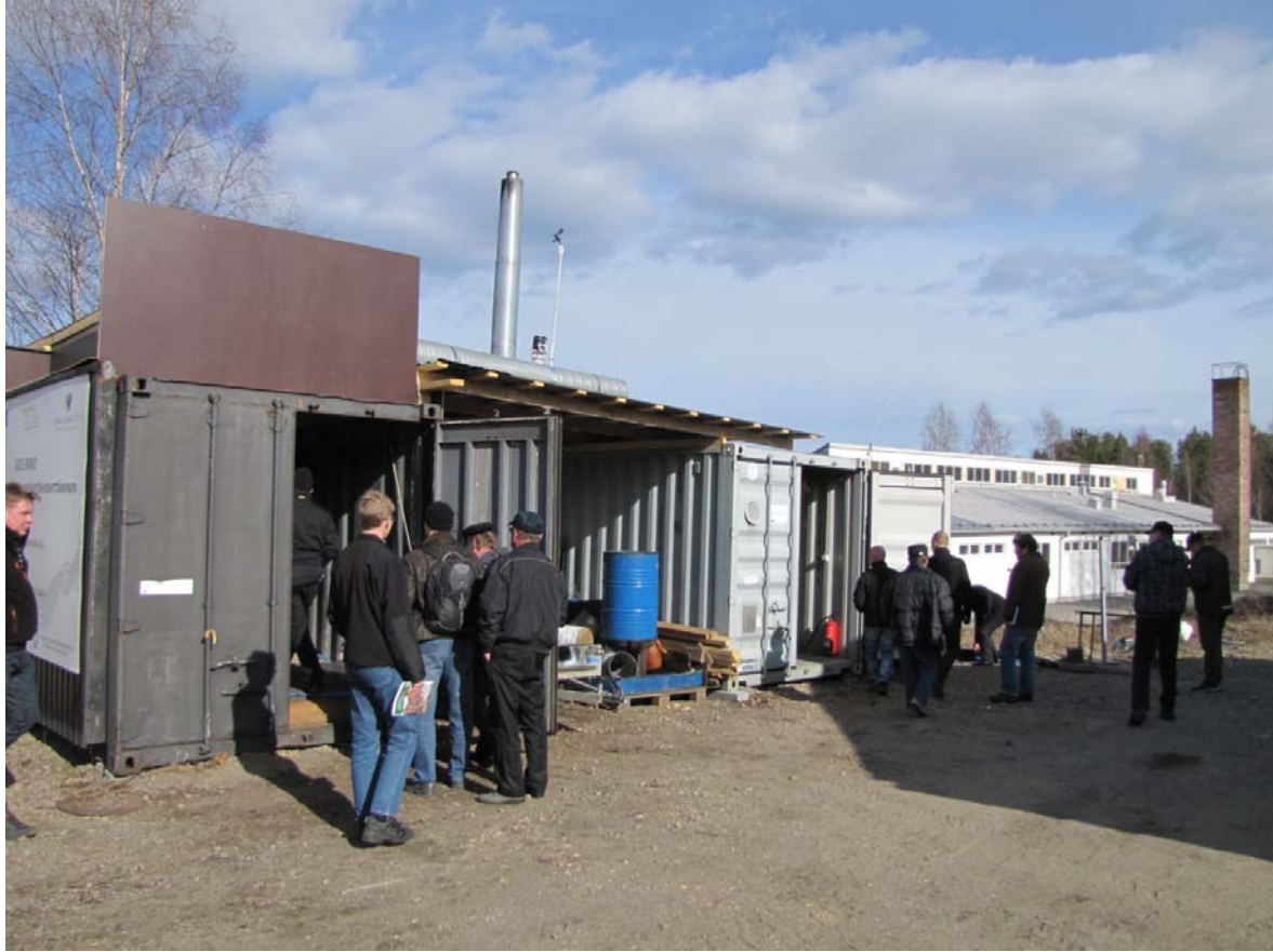
Figure 2. The demonstrated warm air dryer was built into an old freight container (left). A separate 80 kW boiler and control system were placed in another container (right).
