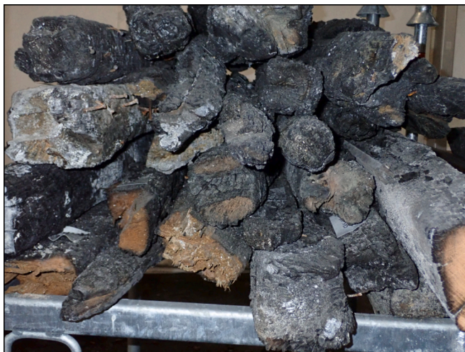
Fig. 1. Example of the carbonisation heterogeneity in the wood beams recovered from the Notre-Dame de Paris cathedral.
