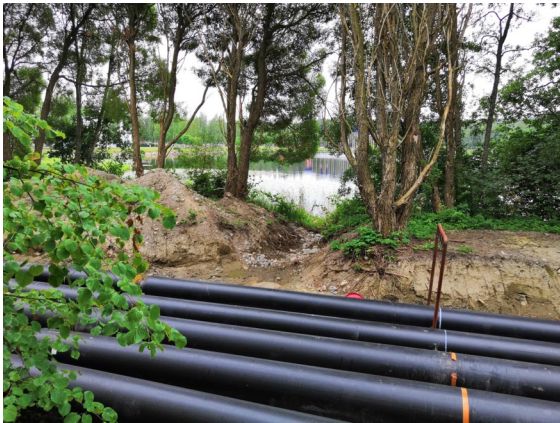
Fig. 3 Construction in progress near the Savilahti bay, district heating and district cooling pipelines installed to a about 160 m long ditch. Photo taken from approximate coordinates 62°53'42.43" N, 27°38'24.47" E, midway along the trench
