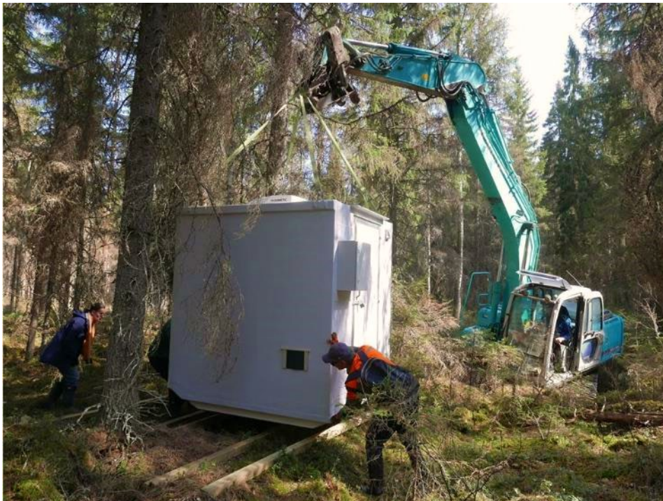
Figure 11. Cabin for the instrumentation. Installation was ongoing in April 2019. Photo: Tuomas Laurila.
