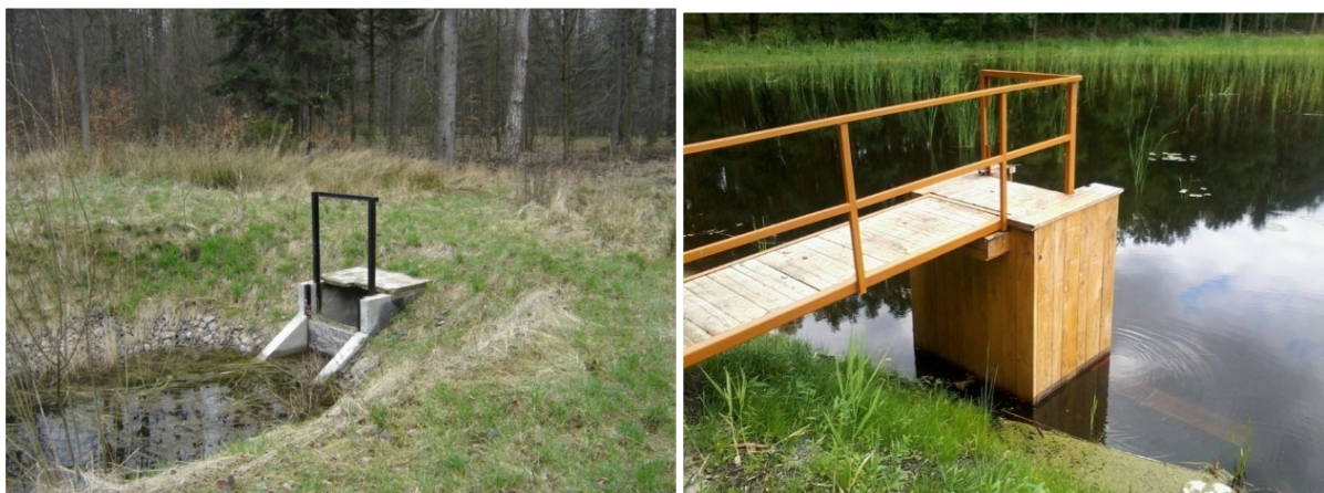
Figure 33. Hydraulic structures controlling water outflow from the reservoirs. Photo by Michał Wróbel.
