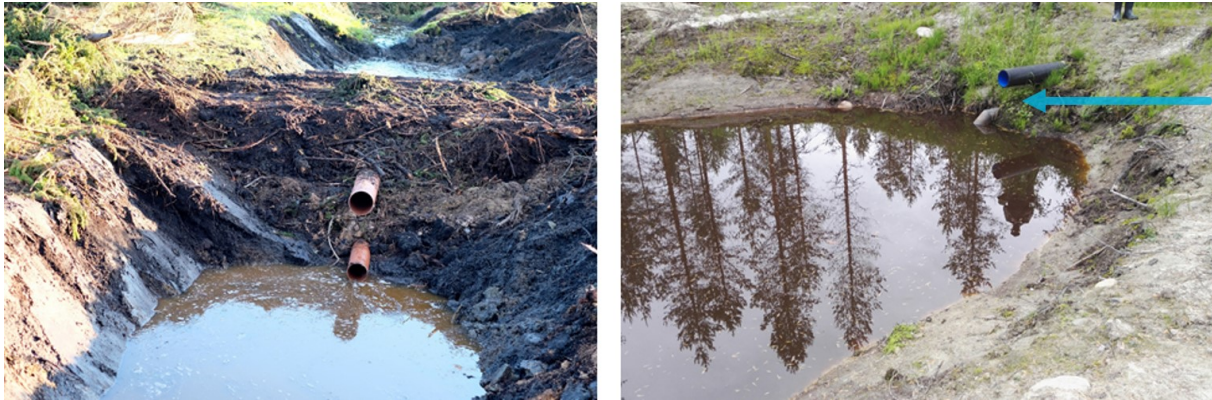
Figure 8. Peak flow control structures at two of the WAMBAF demonstration sites. Note the two visible pipes at the Tobo site in central Sweden (left). Photo by Lars Högbom. Currently, in Vengasoja in central Finland, the upper emergency outflow pipe is visible, the reducer attached to the outflow control pipe is below the water surface (right). Photo by Leena Finér.
