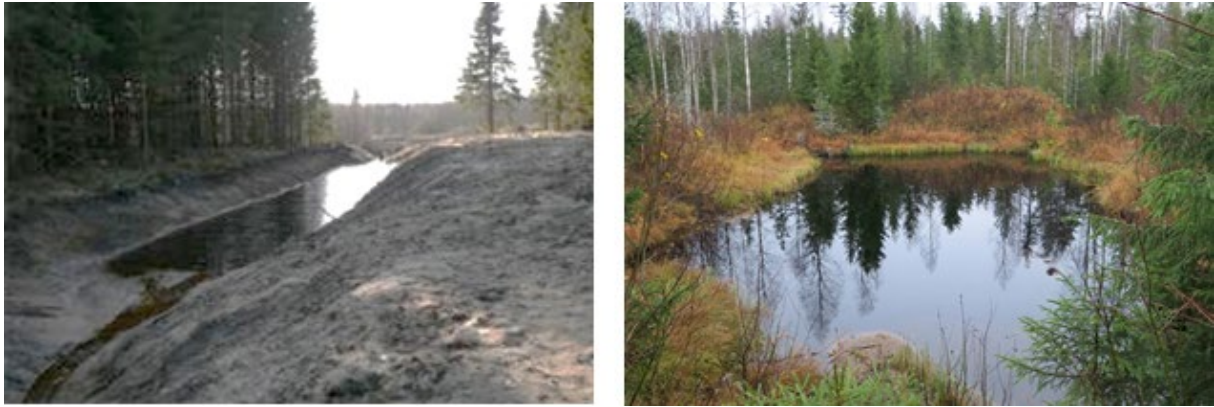
Figure 17. To the left, a newly constructed sedimentation pond in Latvia (photo by Zane Lībiete); to the right, a 20-year-old sedimentation pond in central Finland. Photo by Tommi Tenhola.
