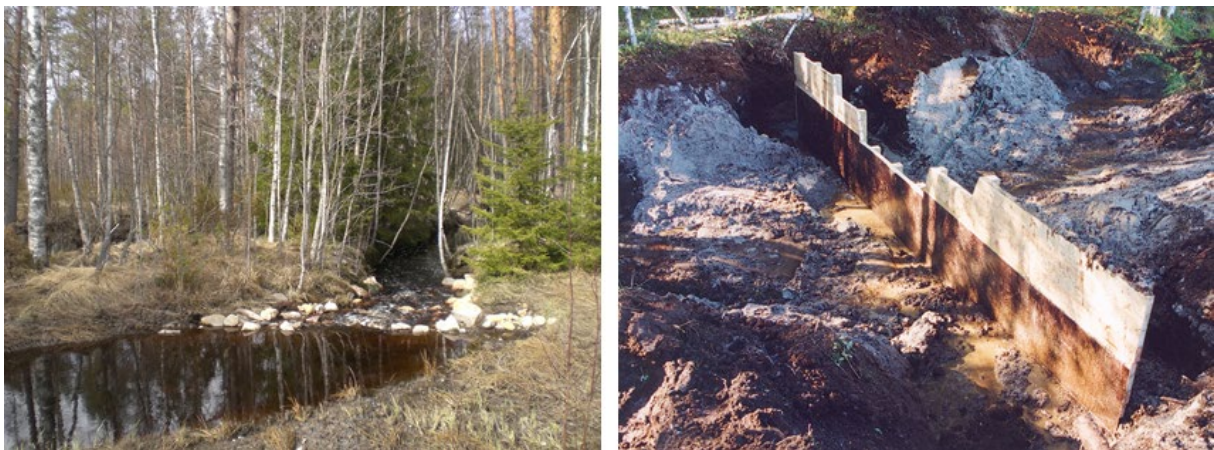
Figure 6. To the left a bottom dam in operation. Photo by Leena Finér. To the right, a supporting wall under construction: it is placed in the middle of the bottom dam across the ditch where the water velocity is expected to be high. Photo by Matti Seppälä.
