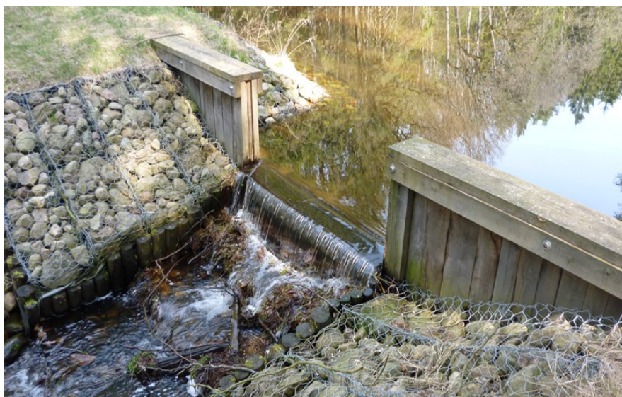
Figure 29. A sluice gate built in a stream to control water level. Photo by Michał Wróbel.
