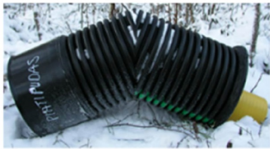
A reducer installed at the end of obstruction barrier
