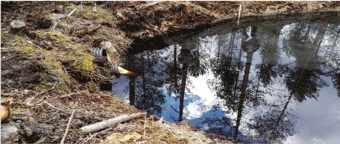
Photo 6. Outlet of a peak flow control structure with two pipes in a drained area located in central Finland. A sedimentation pond has been constructed upstream of the peak flow control structure. Photo Leena Finér.
