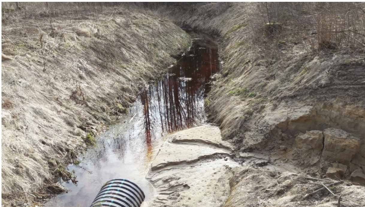
Photo 4. A ditch in Latvia which should not have been cleaned because of the highly erodible soil causing high sediment load to downstream water bodies. Photo Zane Lībieté.
