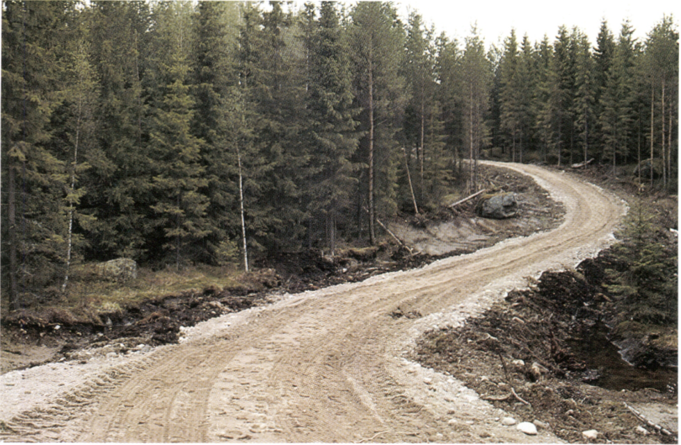
Figure 11. Permanent forest roads serve timber harvesting, silvicultural operations, and the multiple use of forests (Photo Hannu Kalaja).
