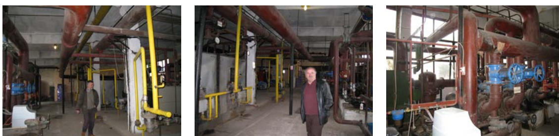
Figure 27. Kos Karoly heating plant; beneficiary: GOSCOM Miercurea Ciuc (Source: GOSCOM and ISPE).
