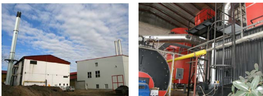
Figure 16. Gheorghieni heating plant.
