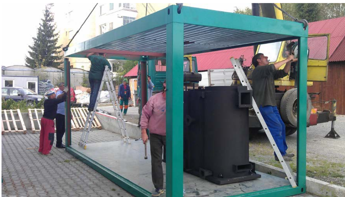
Figure 22. COVIMM Company decided to replace existent heating system with a new biomass boiler (Source: COVIMM).
