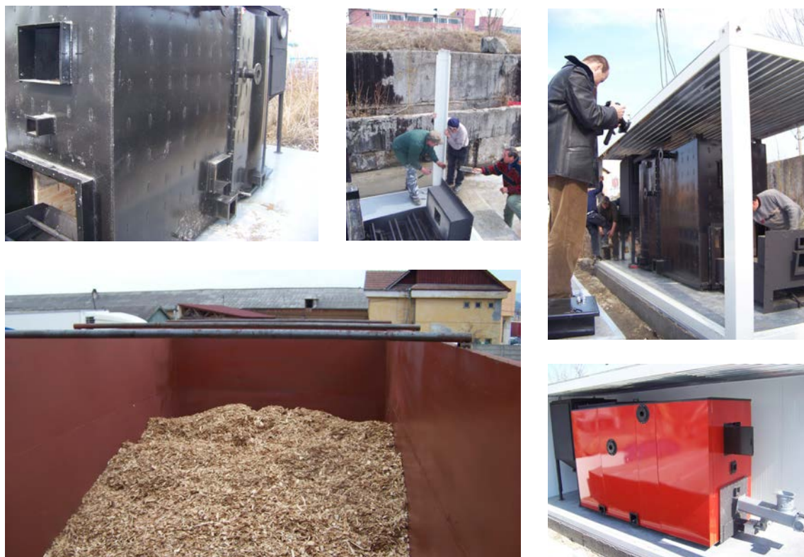
Figure 23. New Bertis Sfantu biomass heating plant (Source: ISPE).
