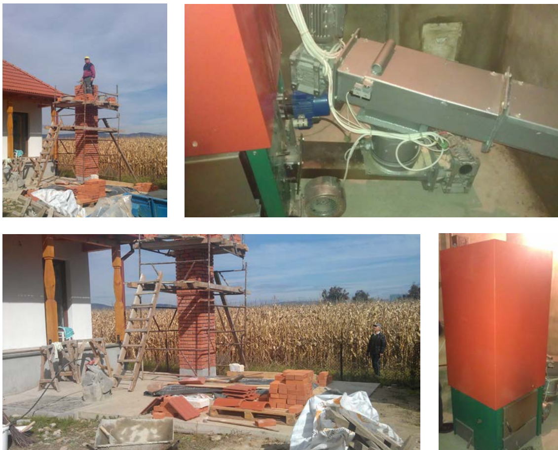
Figure 25. New Kajan Karoly Tg. Secuiesc biomass heating plant (Source: ERPEK IND SRL and ISPE).
