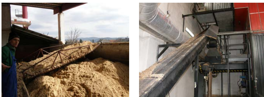
Figure 15. Intorsura Buzaului heating plant.
