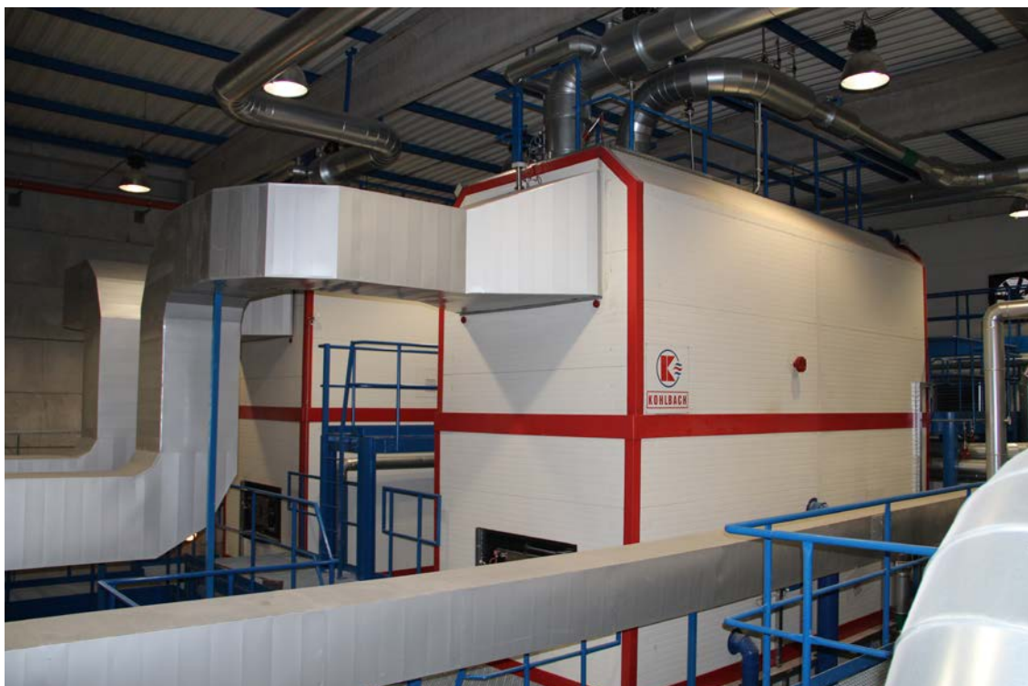
Figure 32. Two biomass boilers (Kohlbach), each with four megawatt thermal output, in the district heating plant Banská Bystrica – Radvaň (Source: DOS-TRADING, Banská Bystrica).
